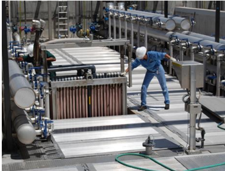
Figure 8. Membrane Cassettes from in a MBR system
