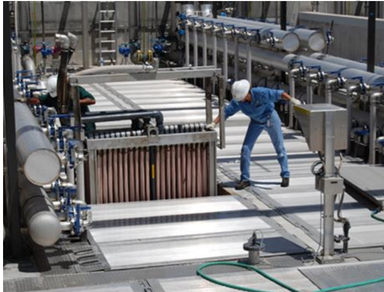
Figure 8-9 Membrane Cassettes from in a MBR system
