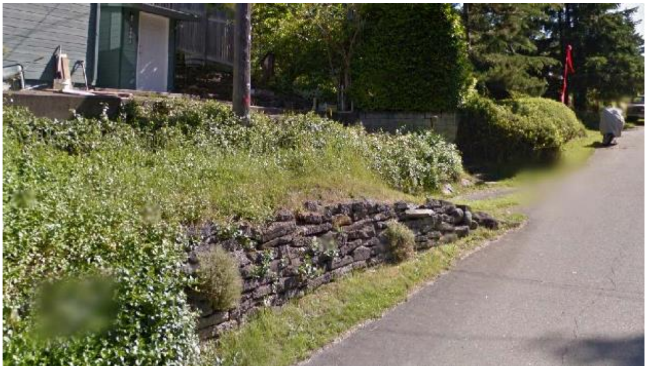
Retaining wall supporting the sloped grade on the north side of Dunsmuir Avenue
