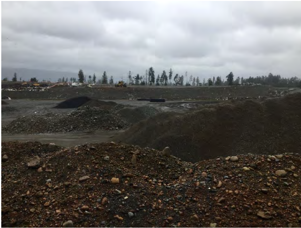
Photo 1. Looking north from the edge of the existing tree stand onto landfill Cell 1. Construction activities show excavated pit and material stockpiles.
