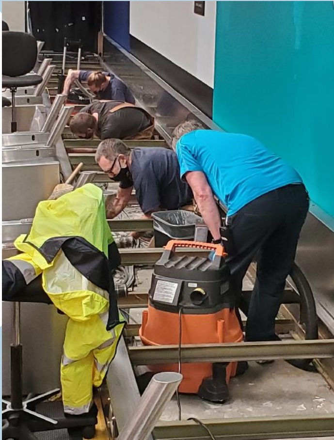
All hands on deck to expedite belt maintenance - CVAC teamwork gets it done.
