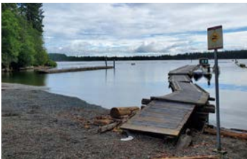
Existing: The dock segment that connects to shore needs to be replaced.
