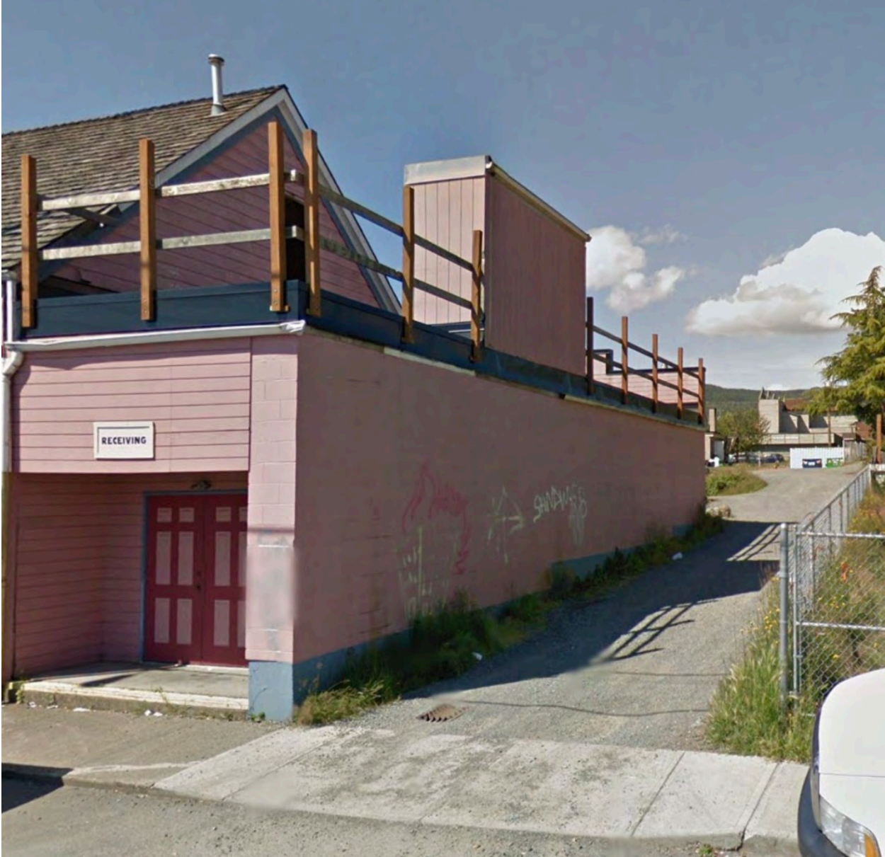
Building, prior to 2013, note the gutters missing from the section closest to Second St.
