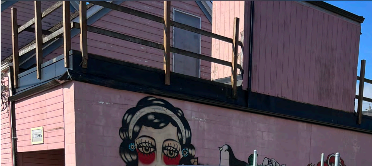
Various states of gutter damage
