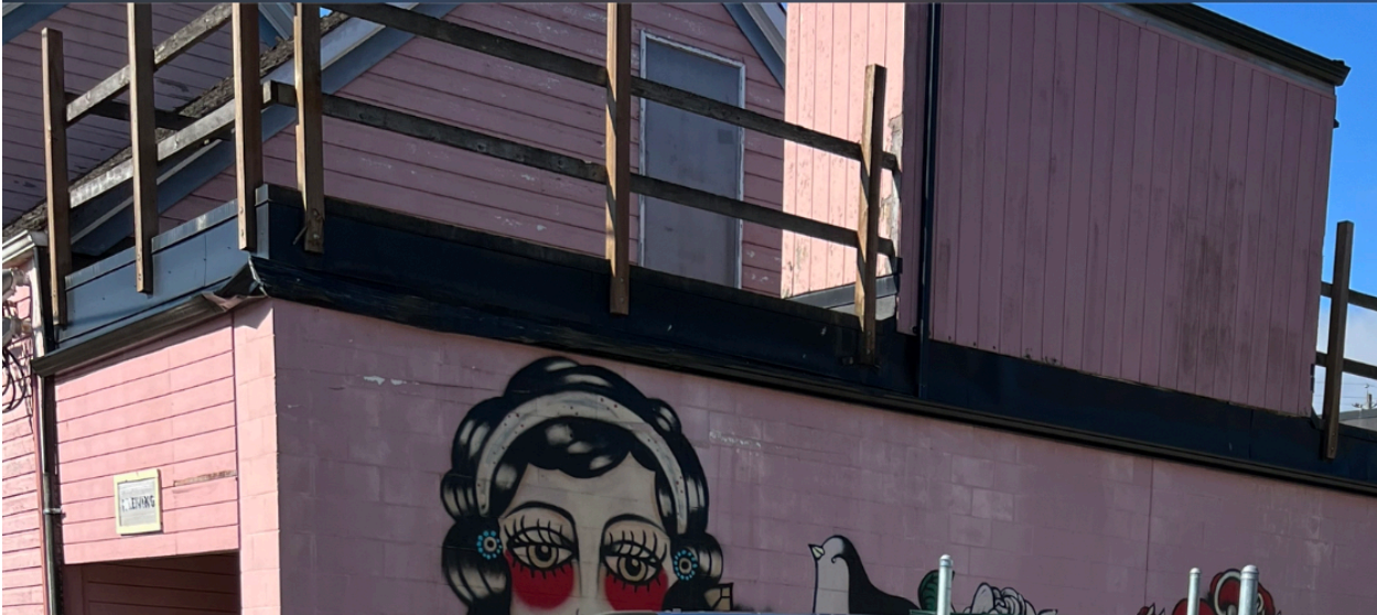
Various states of gutter damage
