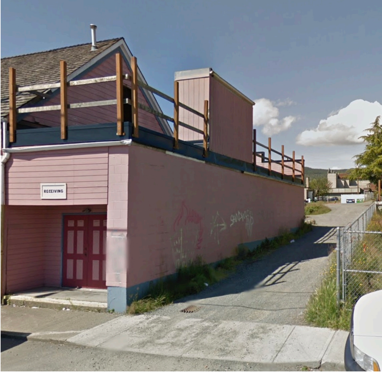
Building, prior to 2013, note the gutters missing from the section closest to Second St.
