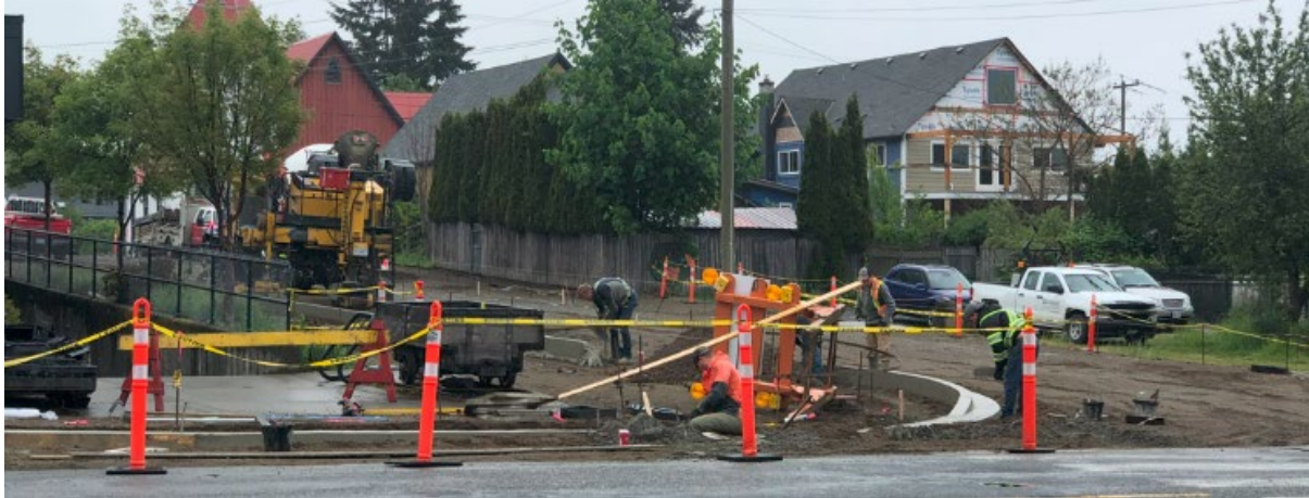
Road and utility construction on First Street between Dunsmuir Avenue and Penrith Avenue
