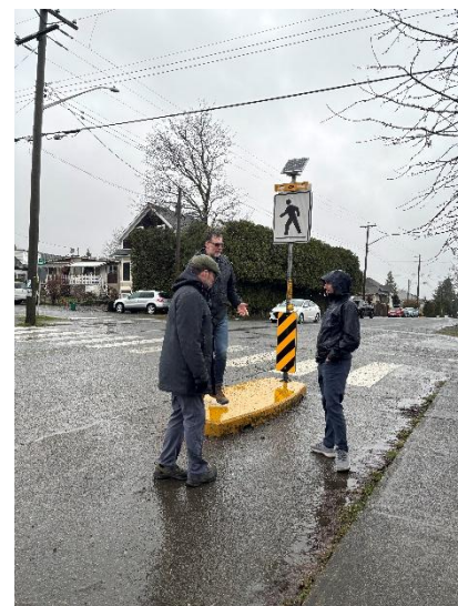
New quick build pedestrian crossing on Fourth Street with traffic calming curbs and rapid rectangular flashing beacons. Committee members are supportive of these types of treatments along the Fourth Street corridor and beyond.
