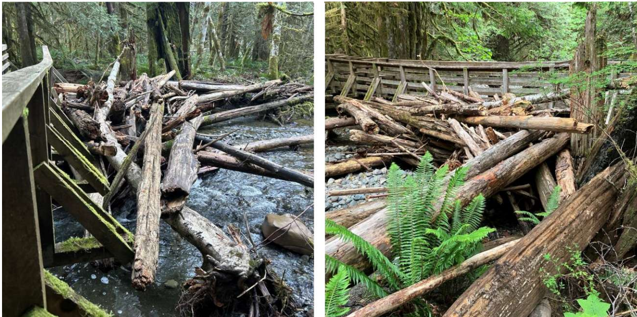
Figure 1.1 Looking at log jam on upstream side of Hai Gai trail bridge. Left photo taken from river left on April 7, 2026. Right photo taken from river right on June 10, 2026.
