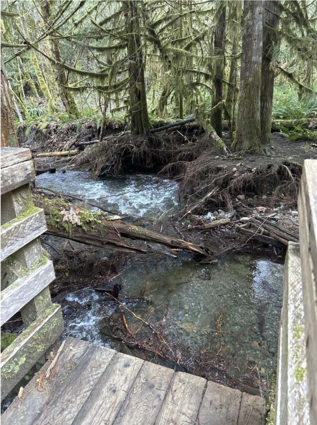
Figure 3.5 Photograph looking downstream at the avulsion channel on April 7, 2026, showing water flowing into the channel from below the bridge.
